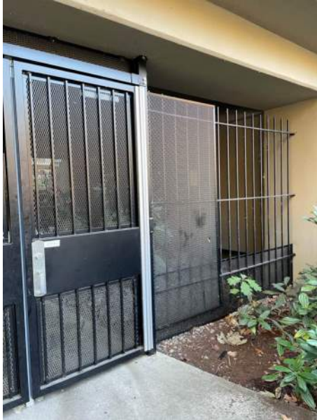
Figure 5: Repaint fence and security panels, Not new gates
